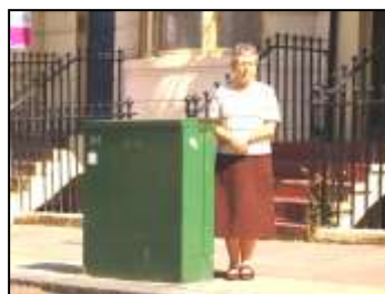
Society member, Suzanne Hinton (5ft 1inch tall), standing next to one of the existing BT boxes.
